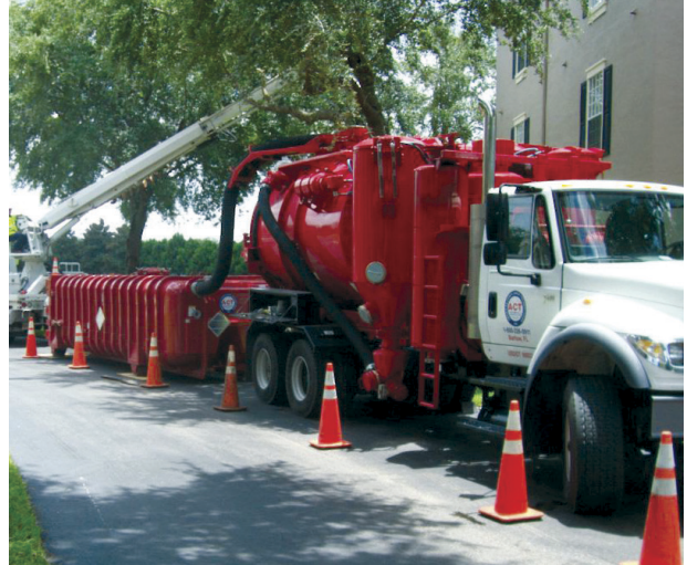
A vacuum truck bypasses its tank and pumps straight into the vacuum container, keeping the vacuum truck at the site working while vacuum containers are filled and hauled away.
